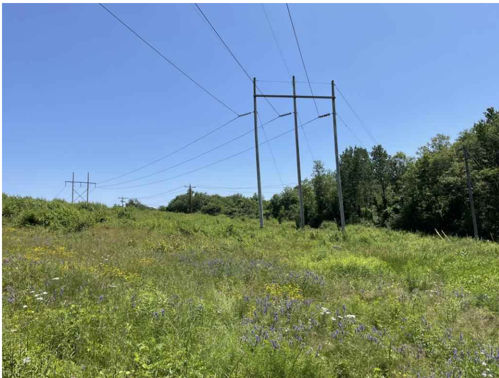
Photograph No. 28: Looking southeast at Structure 4 on the T13 Line ROW off Gosling Road, Portsmouth, NH.
