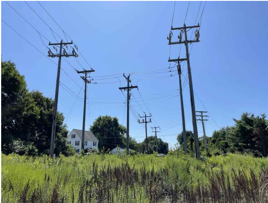
Photograph No. 20: Looking southeast at Structures 72.1 to 72.5 on the 3171 Line ROW off Griffin Road, Portsmouth, NH.
